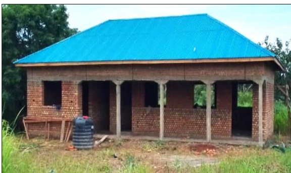
The women's refuge at Tombura begins to take shape. The photo was taken in July 2024.
